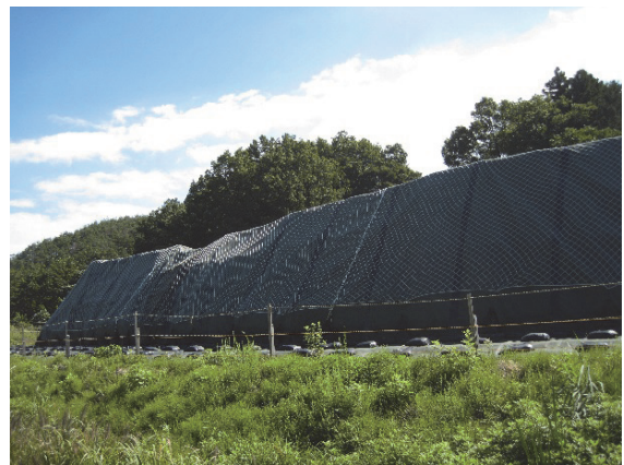
Fig.1 Temporary storage facility of contaminated wastes. The contaminated wastes packed in polyethylene flexible containers were piled up and covered by waterproof rubber sheet.
